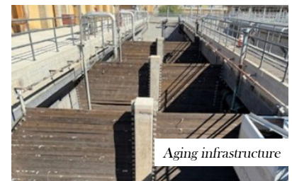
Aeration Tank 1A
